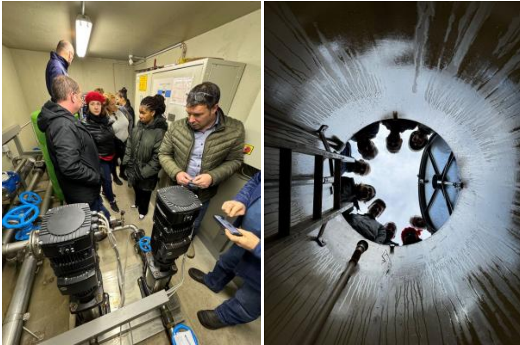
Figure 16: Drinking water cooperative Scheibbsbach: pumping station (left) and view from inside the water reservoir (right).
