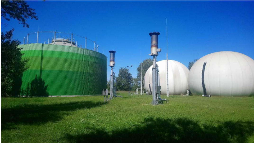
34. Figure: Anaerob digesters and gas sotarage tansk in operation
