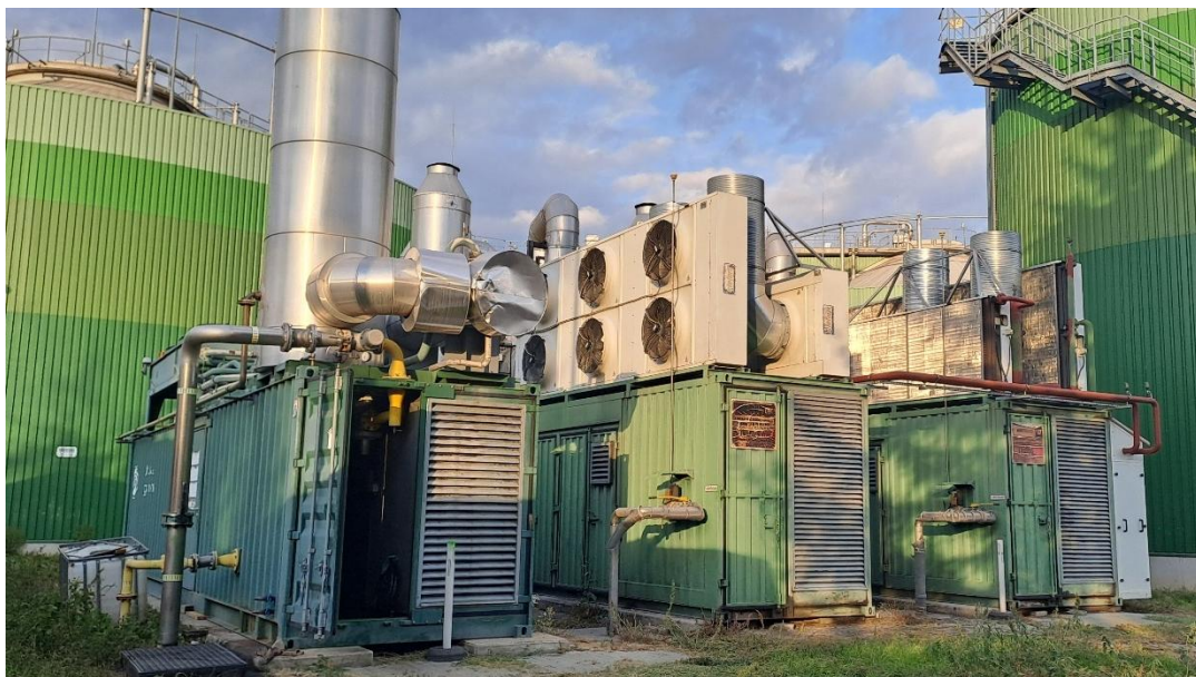
35. Figure: Gas engines utilising biogas
