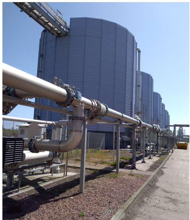
Image 3.2 Biogas generation in anaerobic digesters.
